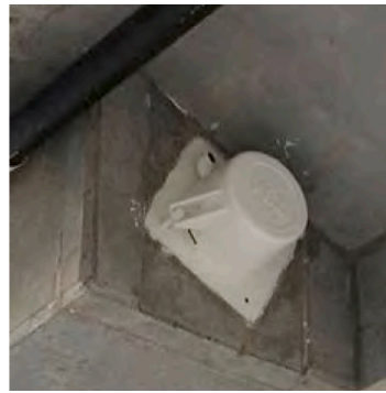
a) Good quality polymer-based end cap at blister of a PT bridge (adapted from [33])
